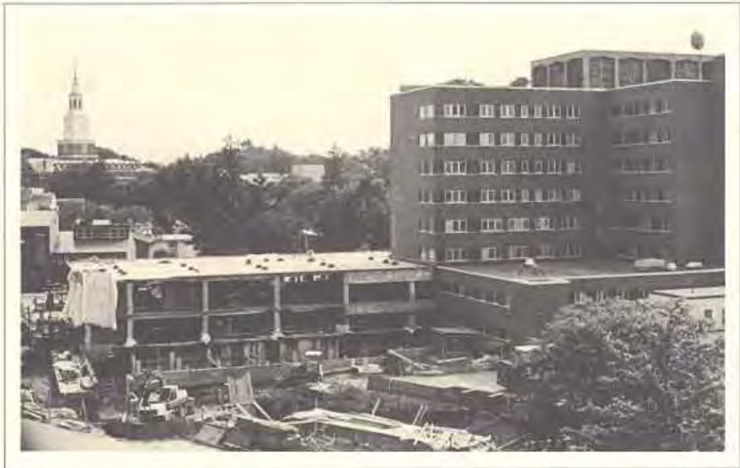
Cancer Center construction—Stage Two. At right is the Mary Hitchcock Memorial Hospital. Beyond, to the left, is the tower of Dartmouth College's Baker Library.
